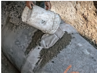
Grout is poured into the diaper into one side and then the other until the diaper is completely full
